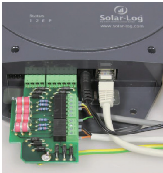
Fig.: Example of overvoltage protection with a Solar-Log 1000
